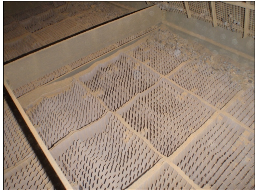
Erosion on East Side (AIG Side)
