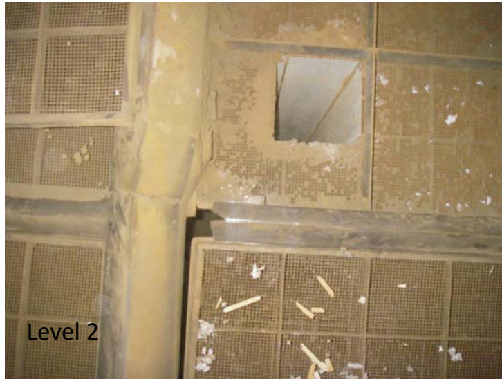
Seal damage (material type)
